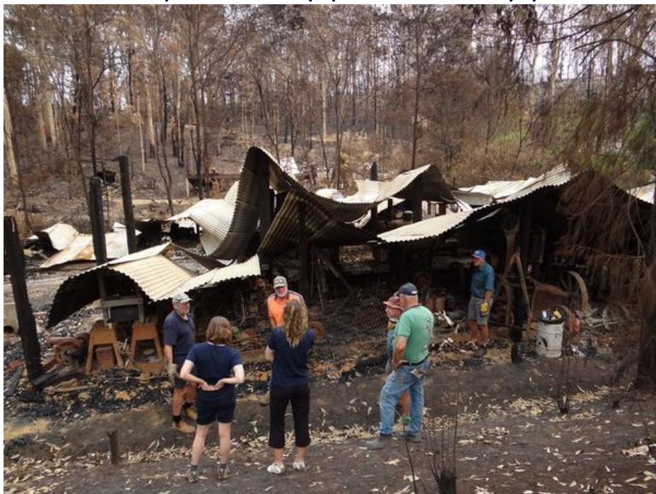
Bimbimbie Fire Damaged remains of MATAMA and EWG shed 2020.
