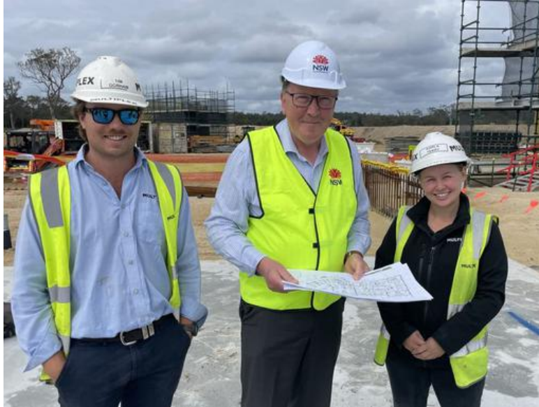
Project Engineer Tim Gorham, Dr Michael Holland and Site Engineer Karla Terry at the ERH site this week.
