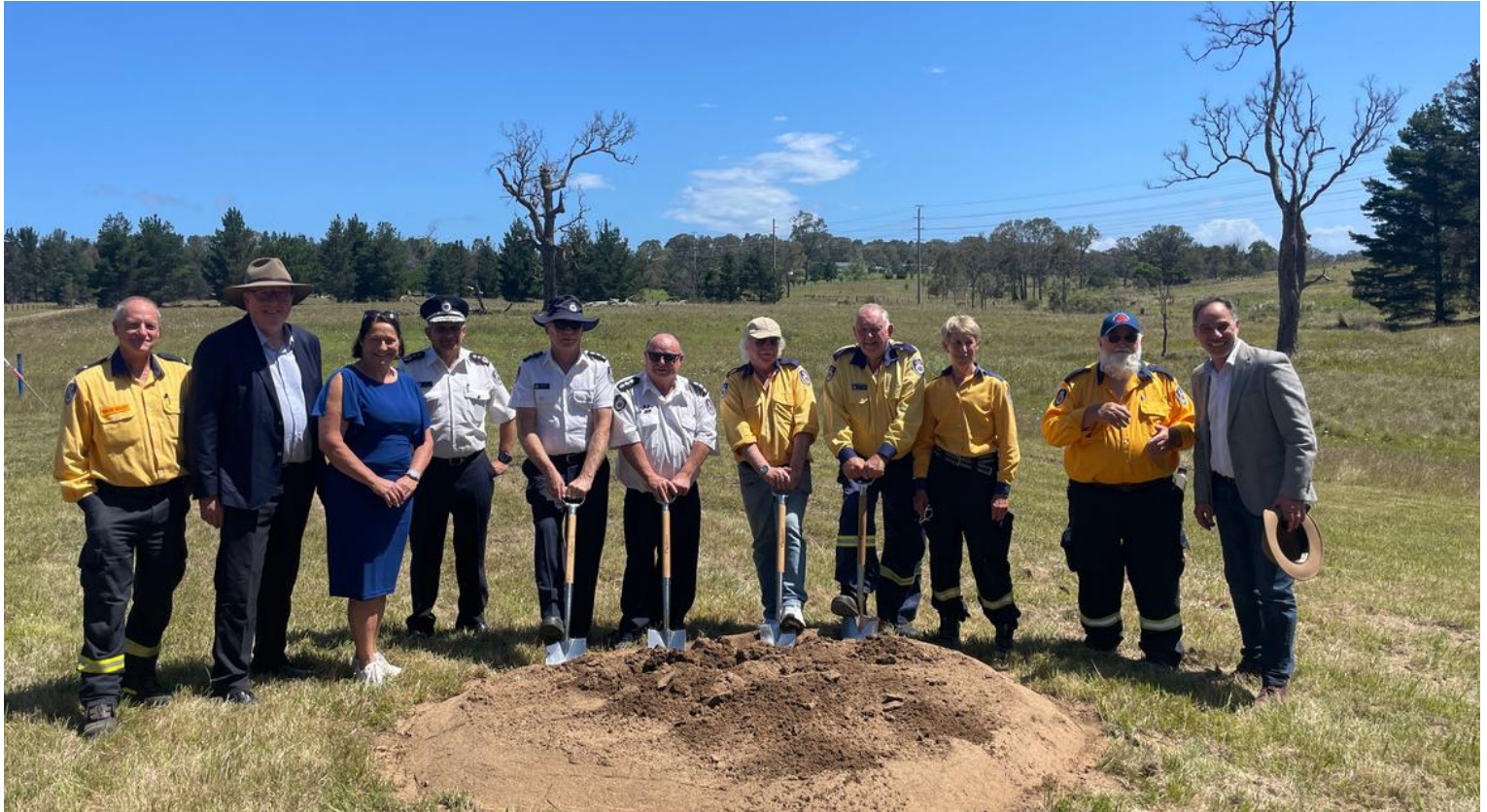
On Tuesday the first sod was turned to mark the beginning of the construction of the Eurobodalla Emergency Services Precinct in Moruya. See p3
