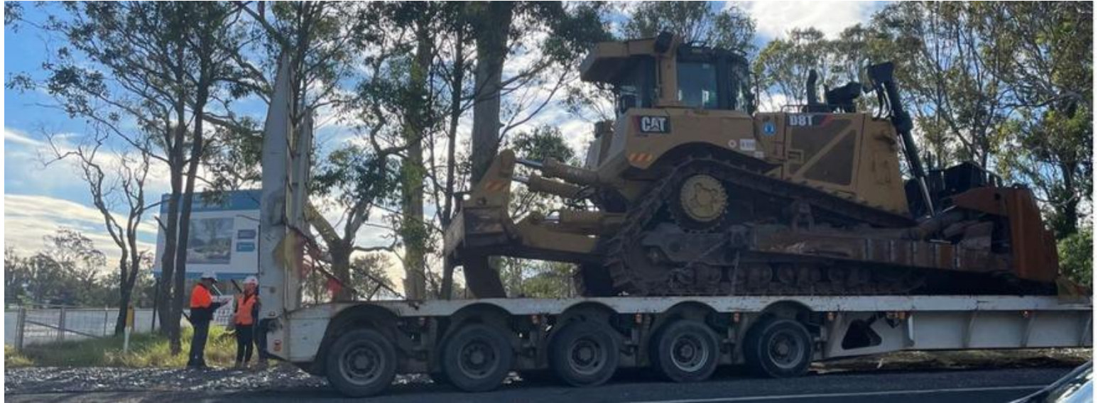
Earthmoving equipment arrives on site at the New Eurobodalla Hospital Photo: SNSWLHD
