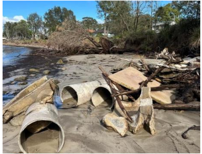
Exposed pipes at Surfside. Photo C Lyttle Facebook
